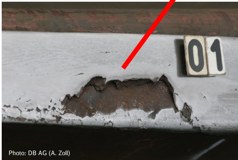
Damage on running surface of crossing nose
